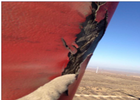
Fig.3 Blade Lightning Strike Damage
