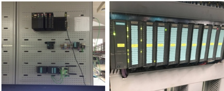
Fig.5 Testing Platform in the Laboratory Environment
